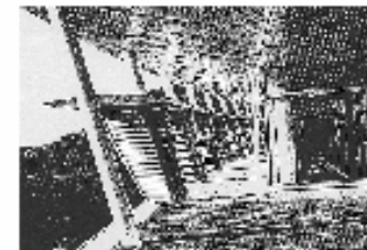
GA04. Institute for Global environmental strategies Light shelves in outside of windows, Japan
